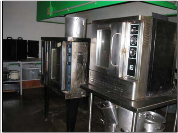
Ovens and Exhaust hood
