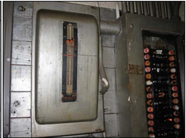
Existing Electric Disconnect and fuse box
