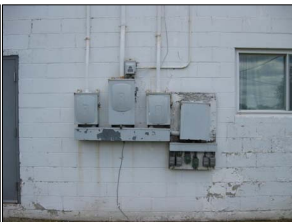
Exterior electrical disconnects
